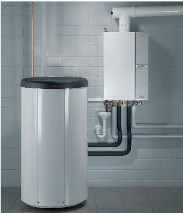
Trinkwassererwärmer WAS neben WTC
